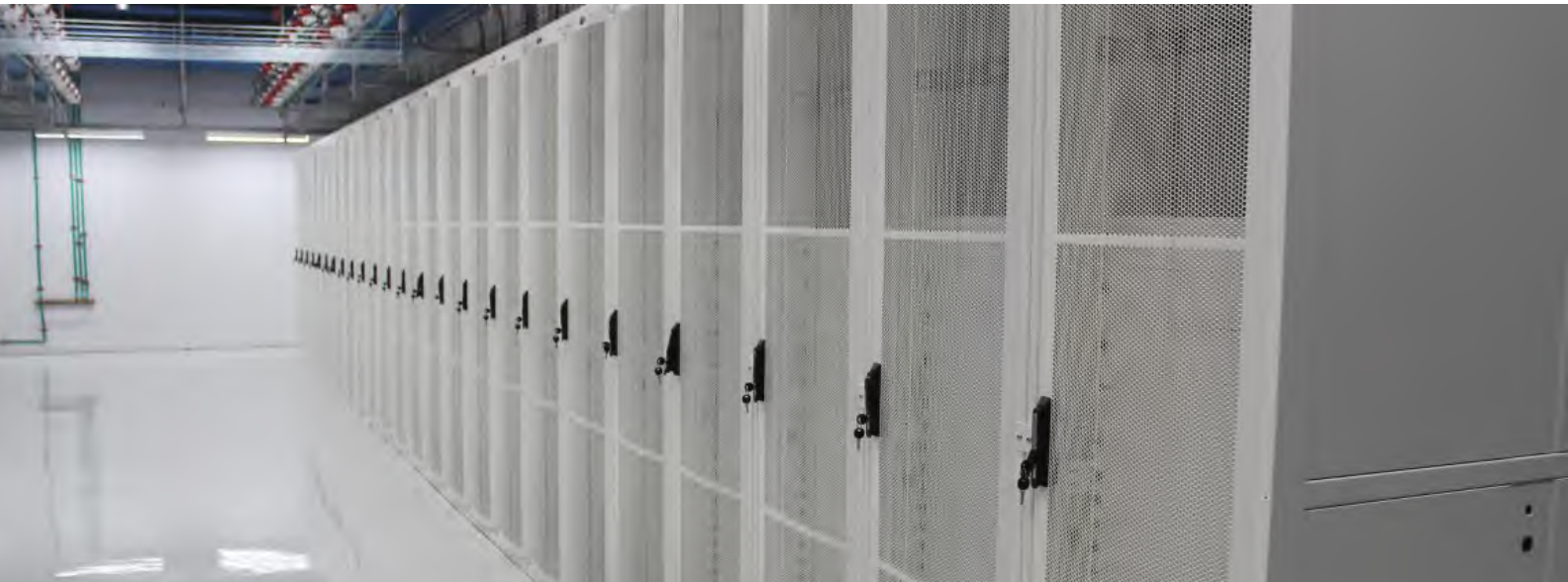
High-density AI-optimised Racks at Larsen & Toubro Vyoma's Data Center
